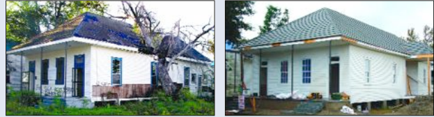
OC's renovation of 4804 Dauphine St. in Holy Cross was the featured "demonstration house" for Restore Media's Traditional Building Show.
